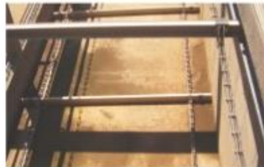
Mechanical Skimming device.
