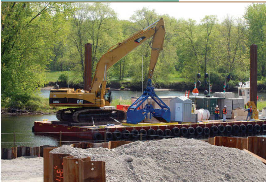
Dredging began in 2009 to remove contaminant sediment from the Hudson River in New York.
